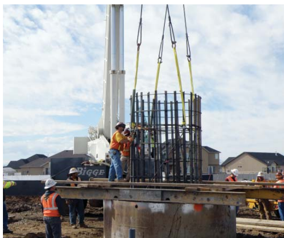
Construction has begun near Layton, Utah on the Populus to Terminal segment of the Energy Gateway transmission project.
