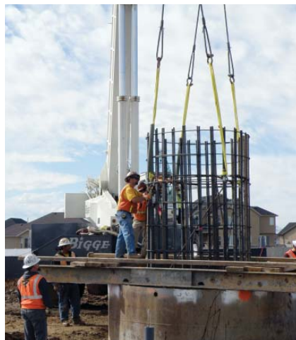
Construction has begun near Layton, Utah on the Populus to Terminal segment of the Energy Gateway transmission project.
