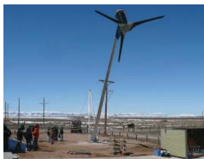
Blue Sky funding helped Casper College, Casper, Wyoming, install a 6-kilowatt wind turbine.
