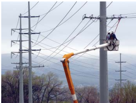
Rocky Mountain Power makes wise investments in the electric system in order to deliver safe and reliable electricity today and into the future.
