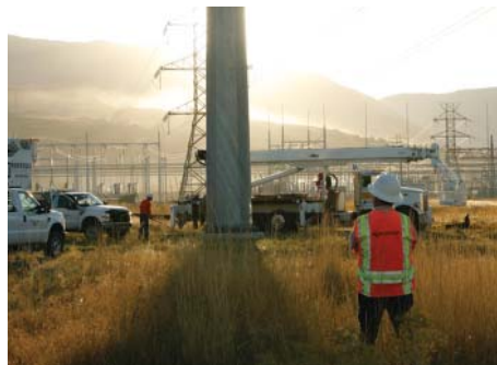
Rocky Mountain Power is building new transmission lines to meet customers' needs.
