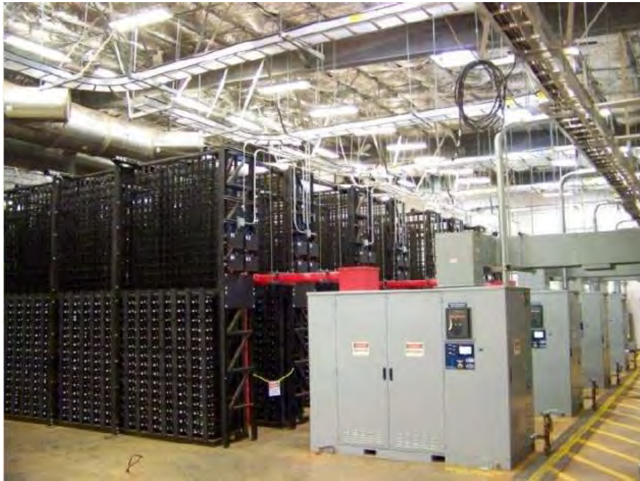
Figure 13 - PowerCell™ Stacks with PCS
