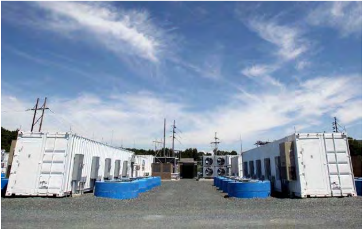
Figure 24 - Flywheel Plant Stephentown, New York
